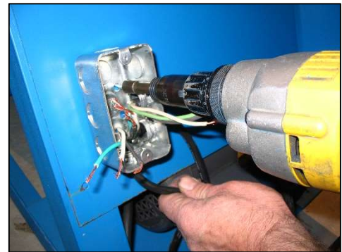
Step 9: Connect wires per schematic. Connect all three ground wires and attach mechanically to box per code. Wire nut all connections.
