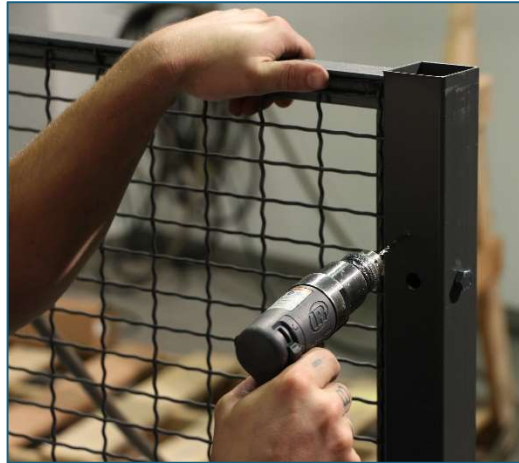
Drill holes for hinges in posts to mount door at desired height.
